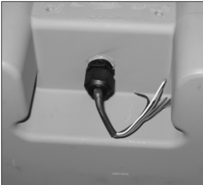
Figure 7.8- Pulse output cable on backside of meter
